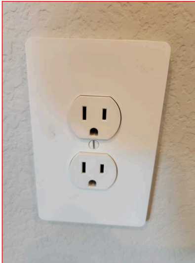
Outlets in home were not tamper resistant.
